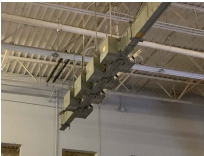
29 - BUS DUCT AND SWITCHES
