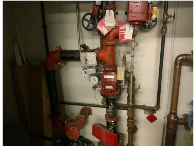
26 - FIRE SUPPRESSION SYSTEM
