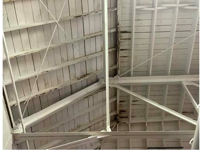
14 - CEILING FINISHES WITH WATER STAINS
