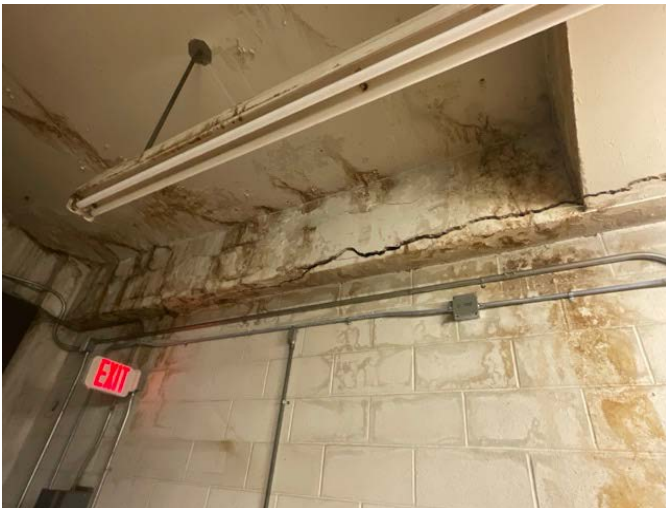
21 - STRUCTURAL CRACK IN BOILER ROOM
