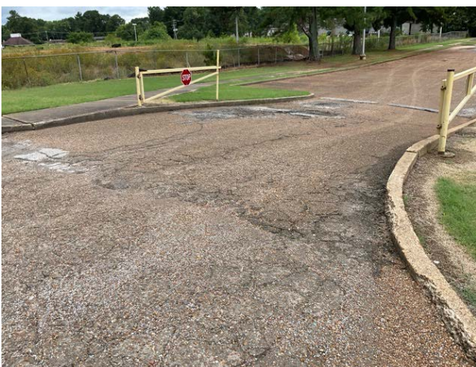
29 - DAMAGED PARKING AREA
